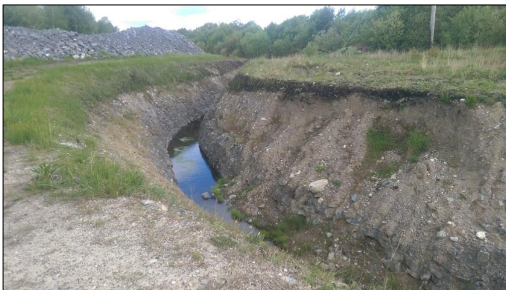
Plate 15.8: View of ditch excavated in the townland of Derryaroge, adjacent to turbine 4, taken from the south.
