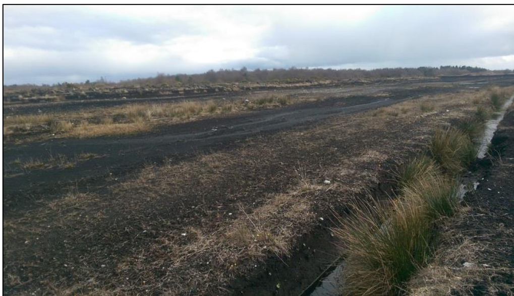
Plate 15.6: View of drains at Turbine 1 and the proposed internal haul road between turbines 1 and 9, taken from the north.
